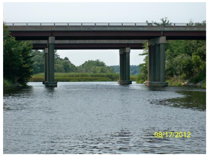
This was taken from the North River going under the Southeast Expressway.
